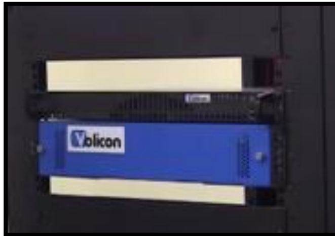
Figure 6.3. Scout Racking - Securing.
